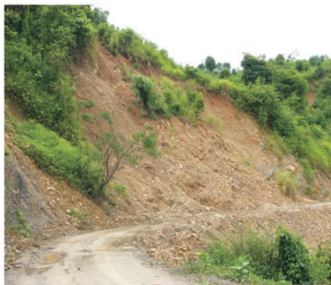
Fig. 4: Debris slide due to unscientific road-cutting
