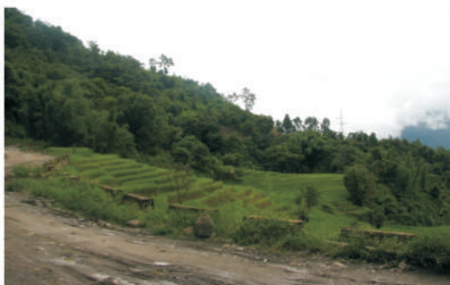
Fig. 5: Road damaged due to water retention for paddy cultivation
