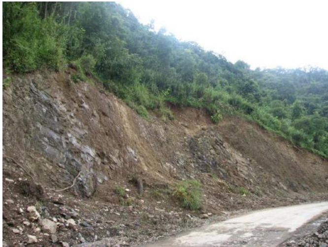
Fig. 2. Weak slope material
