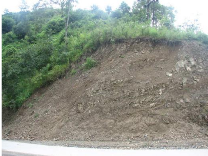
Fig. 5. Weak hill slope
