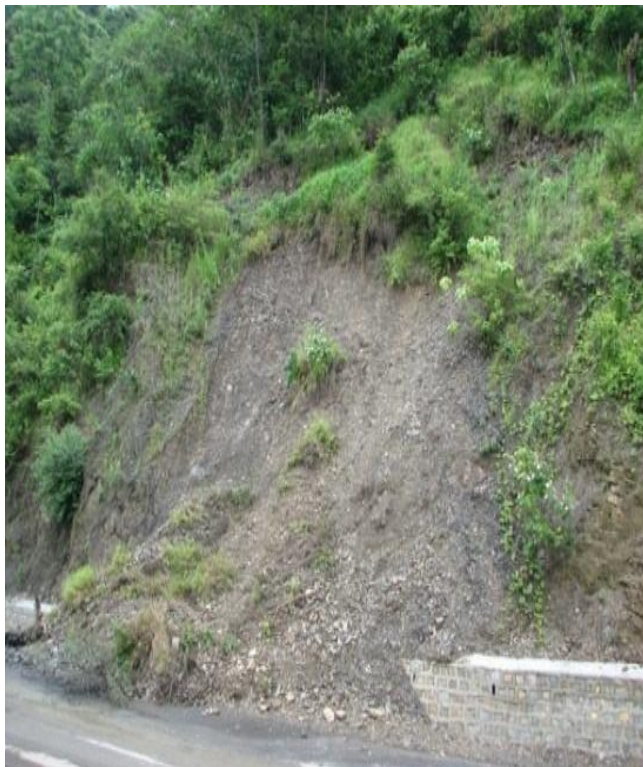
Figure 4. Debris slide in crushed zone
